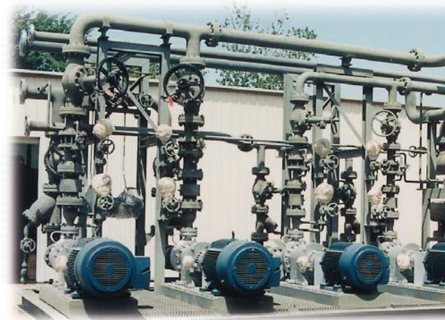
Dual zone 600 kW / 200 kW independently controlled. Included online spare magnetic drive type pumps up to 650° F. located in a petrochemical plant.
