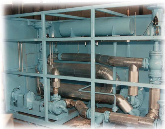
Modified GLOS Hot Oil System with an oversized expansion tank to accommodate the large volume of the customer's system. Temperature control valves were included for flow modulation to multiple zones.
