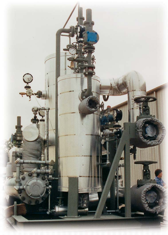
300 kW Hot Oil System designed for Class I, Group D hazardous location with 100% SCR control capable of maintaining the recirculating 600° F. fluid within 1° F. System included vertical expansion tank and vapor recovery tank.
